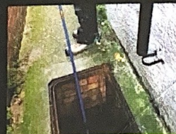
Blocked drains, toilets & sinks
